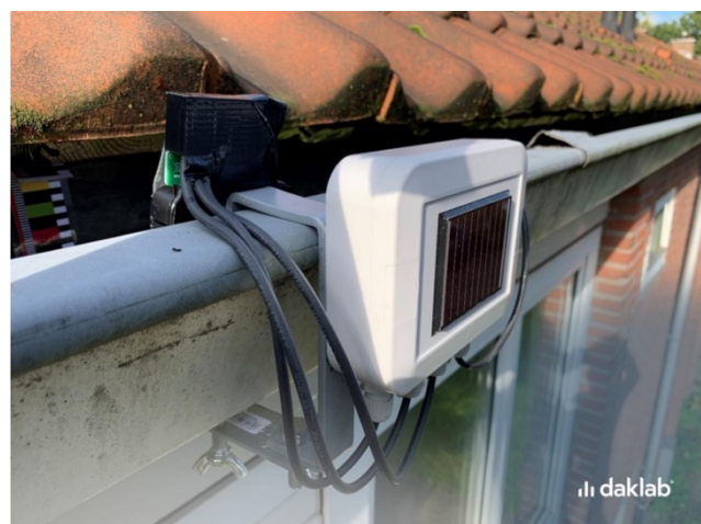
Figuur 56 - Dakgootsensor (Salland Electronics, 2021)
